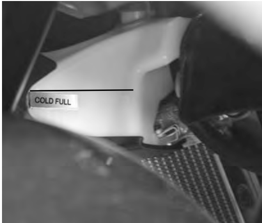
Figure 53. Cold Fill Line.
